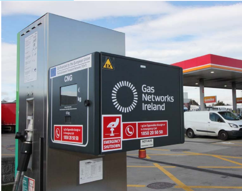
Figure 6-1: Dublin Port CNG Station
